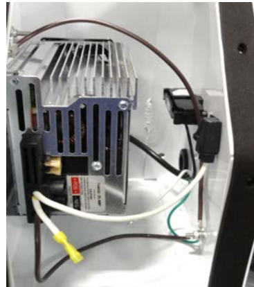
Harness with Relay Removed
